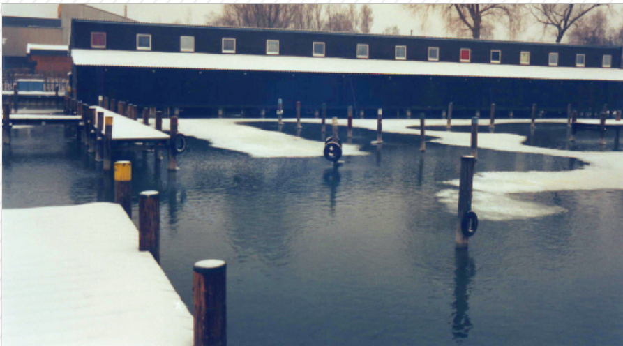
Ice Prevention Plant at -20°
