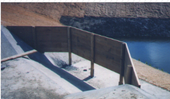
Fixed Diving Baffle Board to protect a spillover weir
