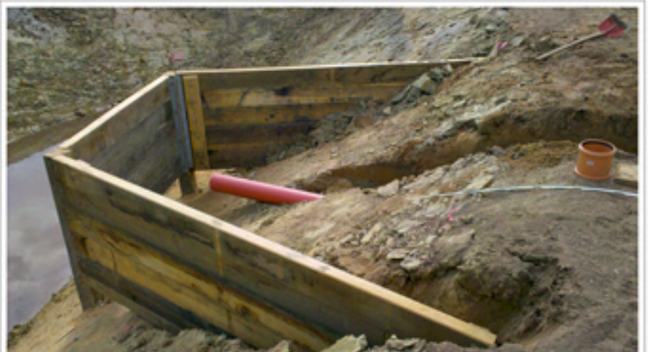
Diving Baffle Board, street water inlet, rainwater retention basin
