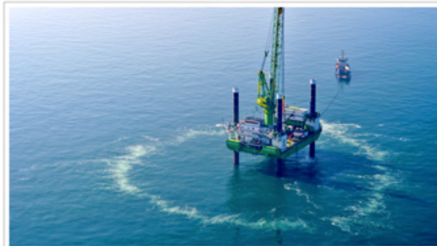
BIG BUBBLE CURTAIN, Baufeld: Borkum West 2 BIG BUBBLE CURTAIN, Construction site: Borkum West 2
