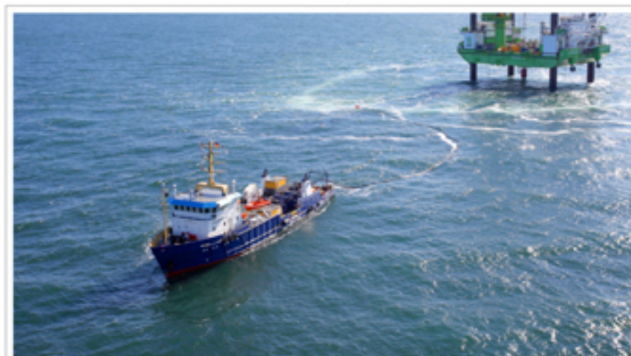
BIG BUBBLE CURTAIN, Baufeld: Borkum West 2 BIG BUBBLE CURTAIN, Construction site: Borkum West 2
